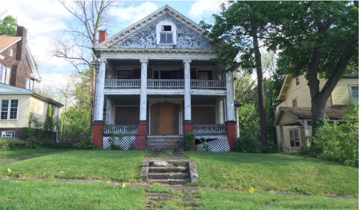
38 Illinois Ave. is an abandoned property that threatens the health and safety of the neighborhood
