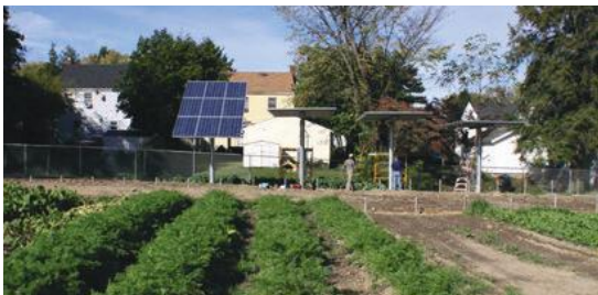
Figure 7.101 - Solar installations at the Iron Roots Urban Farm.
