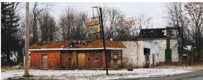
Figure 7.77 - Vacant commercial structures on Hillman Street.
