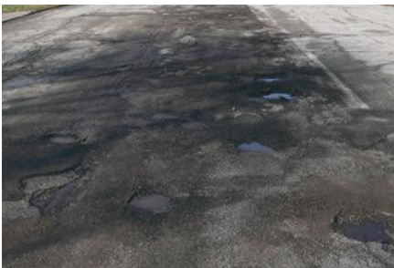
Figure 4.3 - Road conditions on Billingsgate Avenue.
