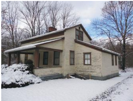
Figure 5.17 - A house in the Idora neighborhood, built in 1850, with severely peeling paint, which is a lead hazard for neighborhood youth.
