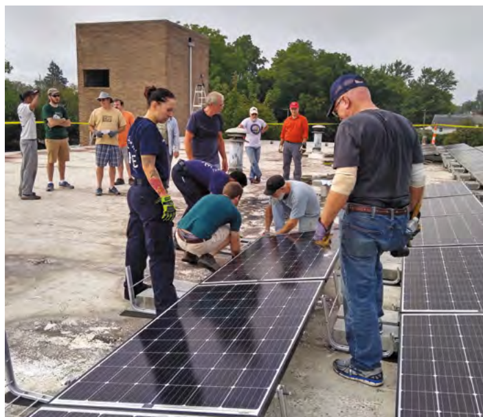
SolarYpsi volunteers install solar panels atop a fire station in Ypsilanti, Michigan. Source: ESAL.
